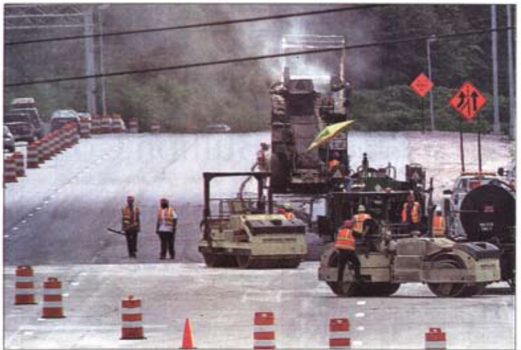
Workers pave part of Interstate 40 in downtown Knoxville in this July 2001 photo. The high price of asphalt means state and local governments are pursuing fewer road projects these days. Bruce Wuethrich, senior director of engineering and public works for Knox County, said the county has not had to sacrifice capital projects — the building of new roads or major reconstruction projects that generally cost more than $50,000. Instead, it has scaled back maintenance projects in subdivisions.
